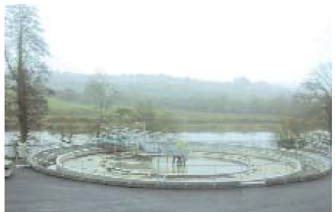
Graiguenamanagh Wastewater Treatment Plant
