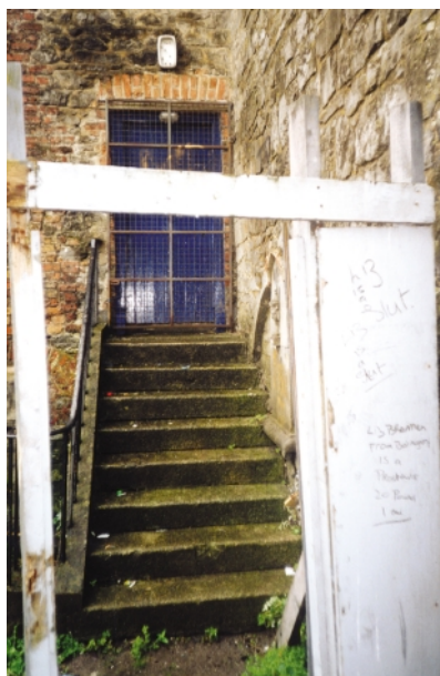
Plate 30: Neglected rear entrance doorway
