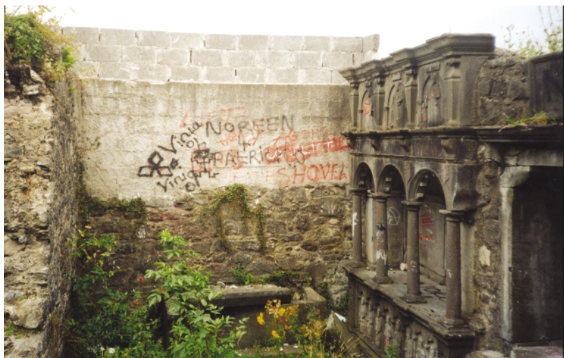
Plate 29: Damage caused as a result of cleaning off graffiti
