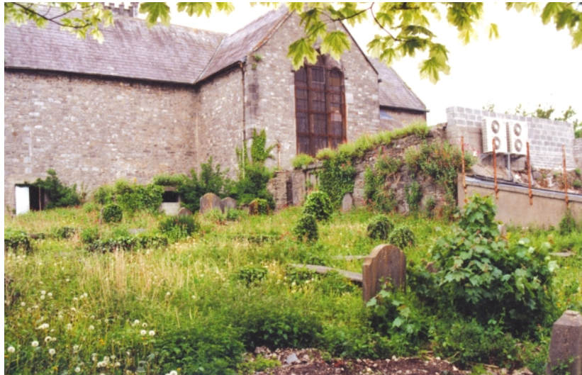
Plate 21: The derelict Almshouse
