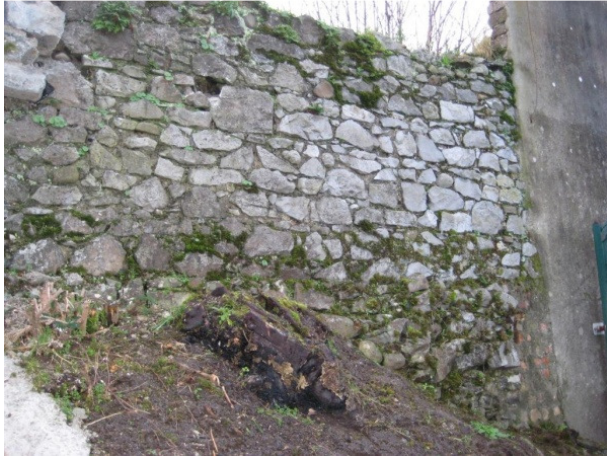
The section of north curtain wall before work started. Works undertaken included removal of vegetation, repair of wall top and some repointing.
