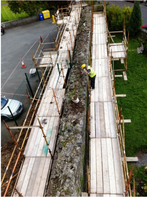
View of the east curtain wall scaffolded and ready to commence work.
