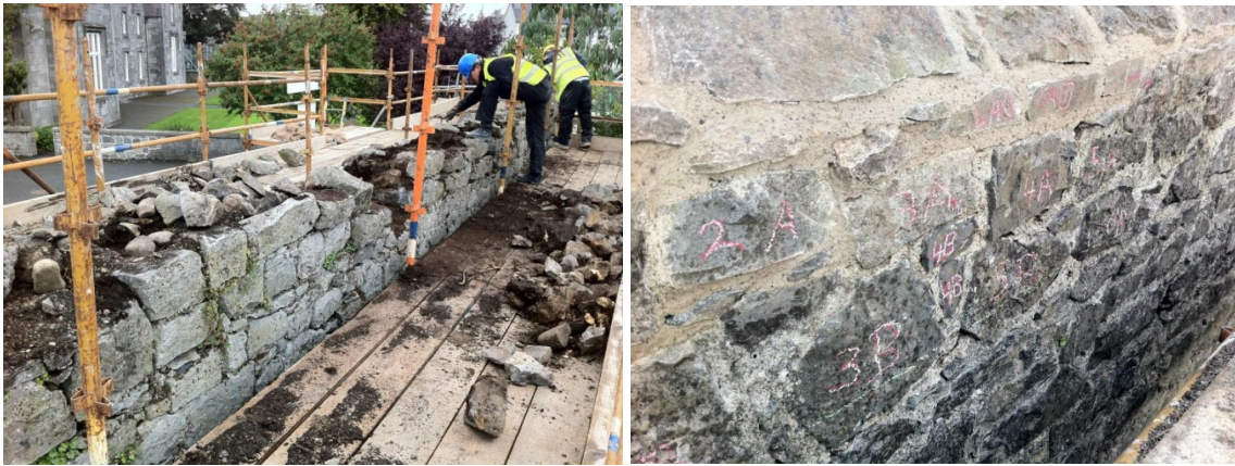
The wall was surveyed. Stones were numbered and removed in small batches before being rebuilt.
