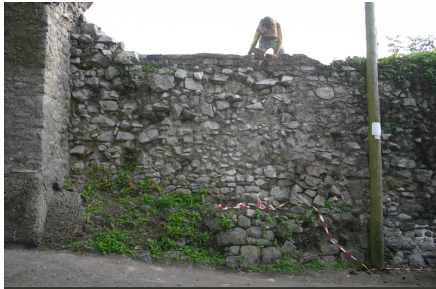
Surveyed in September 2008 indicates further deterioration and significant loss of fabric.
